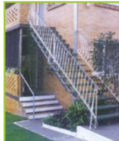
Paint on edge of stairs (on the riser)
